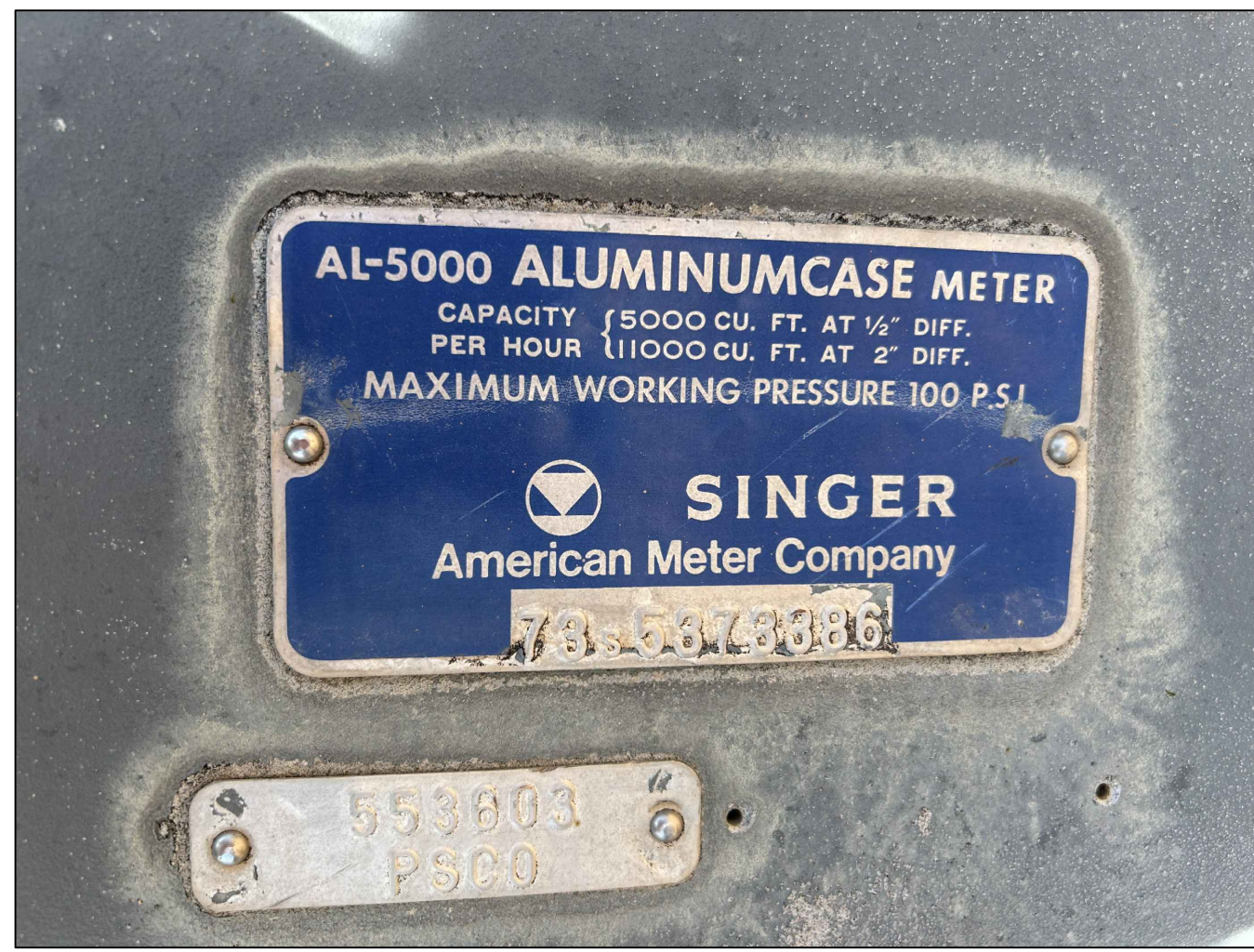
EXISTING GAS METER NAMEPLATE INFORMATION
